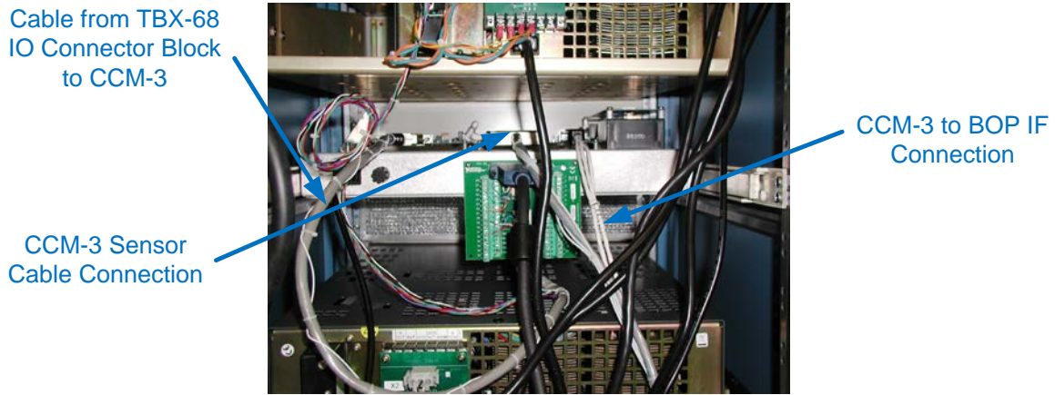
Figure 5 Rack rear view details
